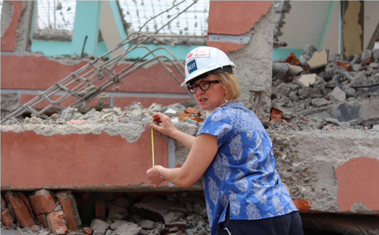
Svetlana taking measurements of a collapsed home in Kathmandu. Seismic design concepts were not incorporated in many concrete buildings. The size of the beam is significantly larger than the column in this frame building, violating seismic design rule. (Photo credit: Bishnu Pandey)
